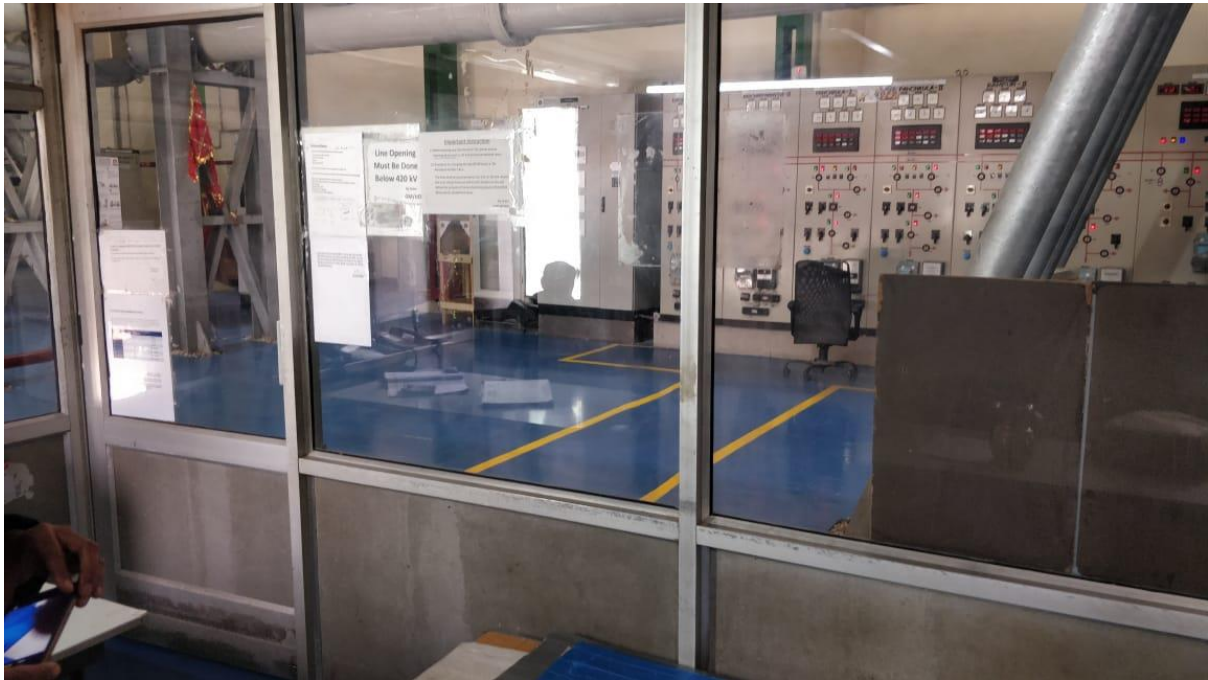
Figure-1: Monitoring Room and Electric Panel of the Power Plant
