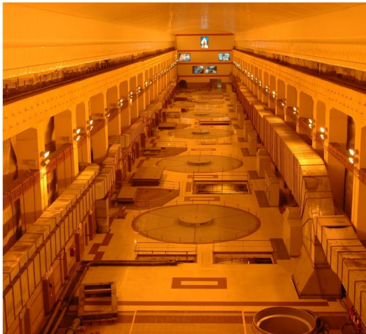
Power House of 1500 MW Nathpa Jhakri Hydro Power Station, Jhakri (HP)
